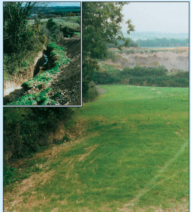
Rehabilitated site of exploration trench beside hedgerow in foreground, near Inishannon, Co. Cork. Inset: open trench.
